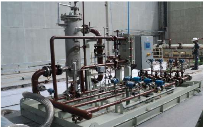
Portable Lube Oil System (SIEMENS)
