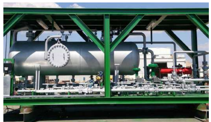
Three Phase Separator Skid – (CCED, Oman)
