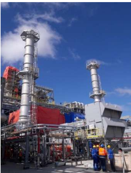
Gas Turbine Exhaust System (MAN Diesel & Turbo, Germany)
