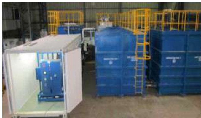
Containerized Skid (SUEZ)
