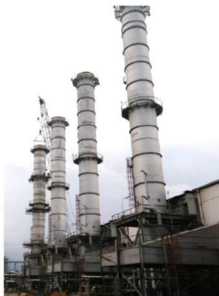
Gas Turbine Exhaust System (Indorama, Nigeria)
